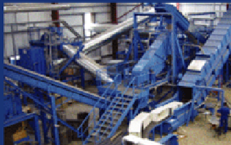
Recycling of cooling and freezing equipment
